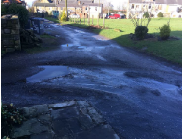
Photograph 3 – damaged caused by the water run-off and tractor to the un-adopted lane to the rear of N o s 351 and 355 Haslingden Road.
